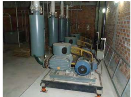
Wastewater Treatment Facilities in Aeon Mall
