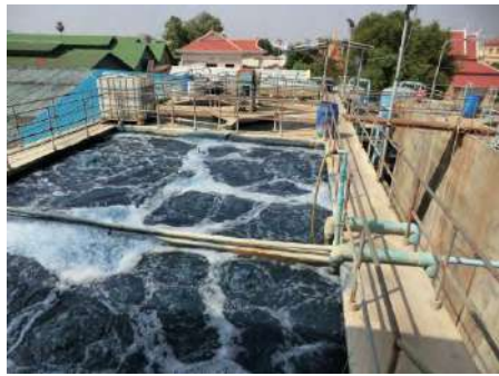
Wastewater Treatment Facilities in Dye House
