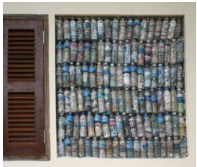
The Eco Blocks are tied together to create blocks that build up the wall which is then covered with chicken net.
