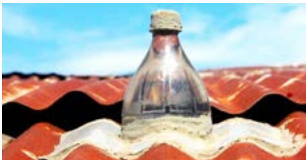
Solar bottle light in metal roof
