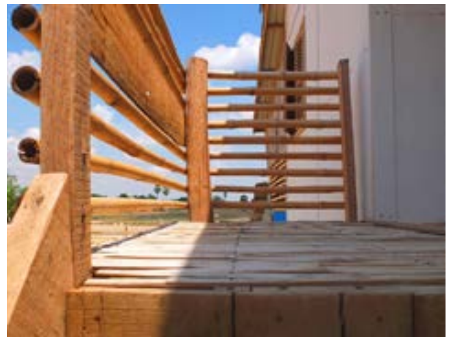
Site specific wall and floor materials reduce the overall cost and carbon footprint
