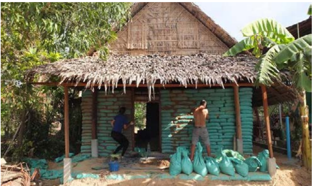
Mixing traditional Khmer features of the palm tree leaf weave roof with the earthbag technique
