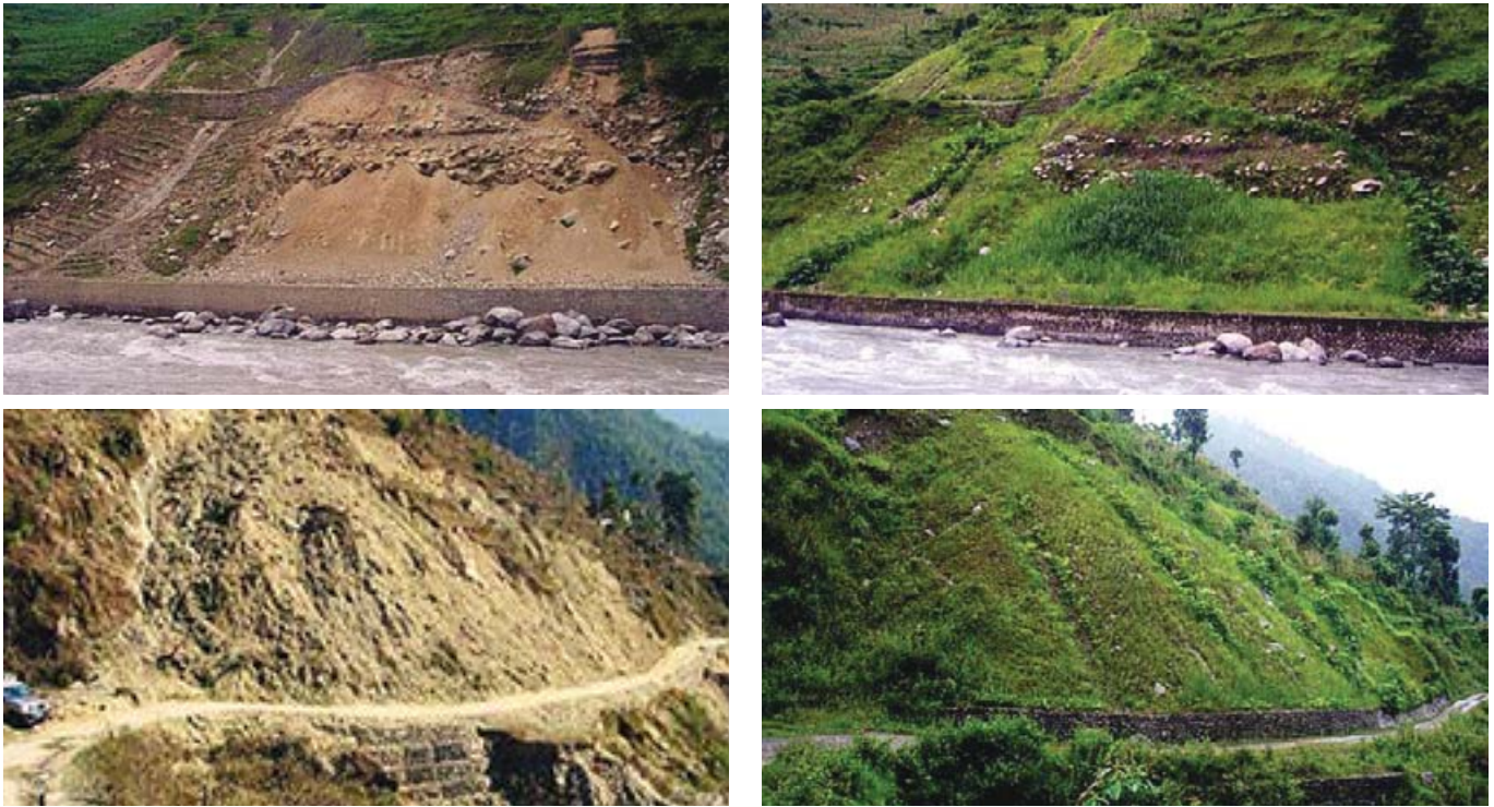
Slope stabilization methods were used for the Balephi landslide Source: Nepal District Road Support Program. www.flickr.com
