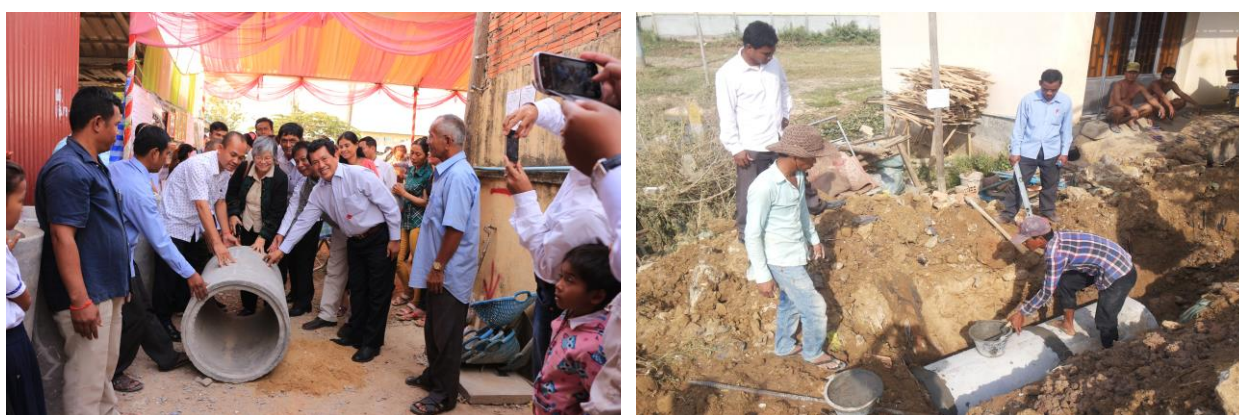
Drainage installment in low income community in the outskirts of Phnom Penh
