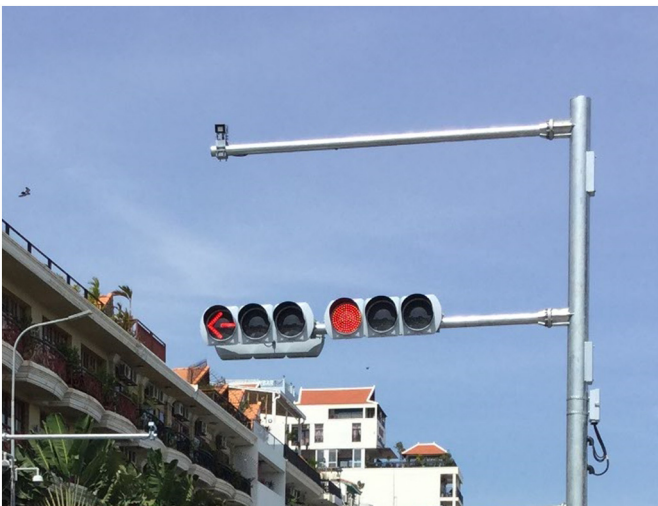
Fig. 10. Newly installed signal with video vehicle detector above.
