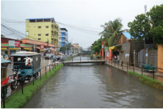
Figure 19: The Street 105 sewage canal approaches overflow during a heavy rain mixing sewage, gray water, and trash with storm water.
