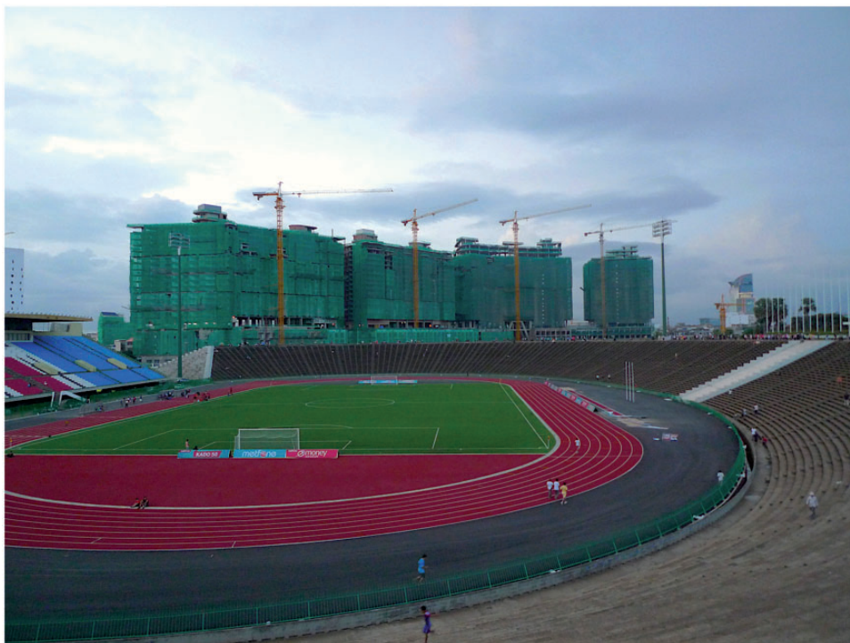
Figure 1. The National Stadium and the Olympia City project under construction in 2015 in the background.
