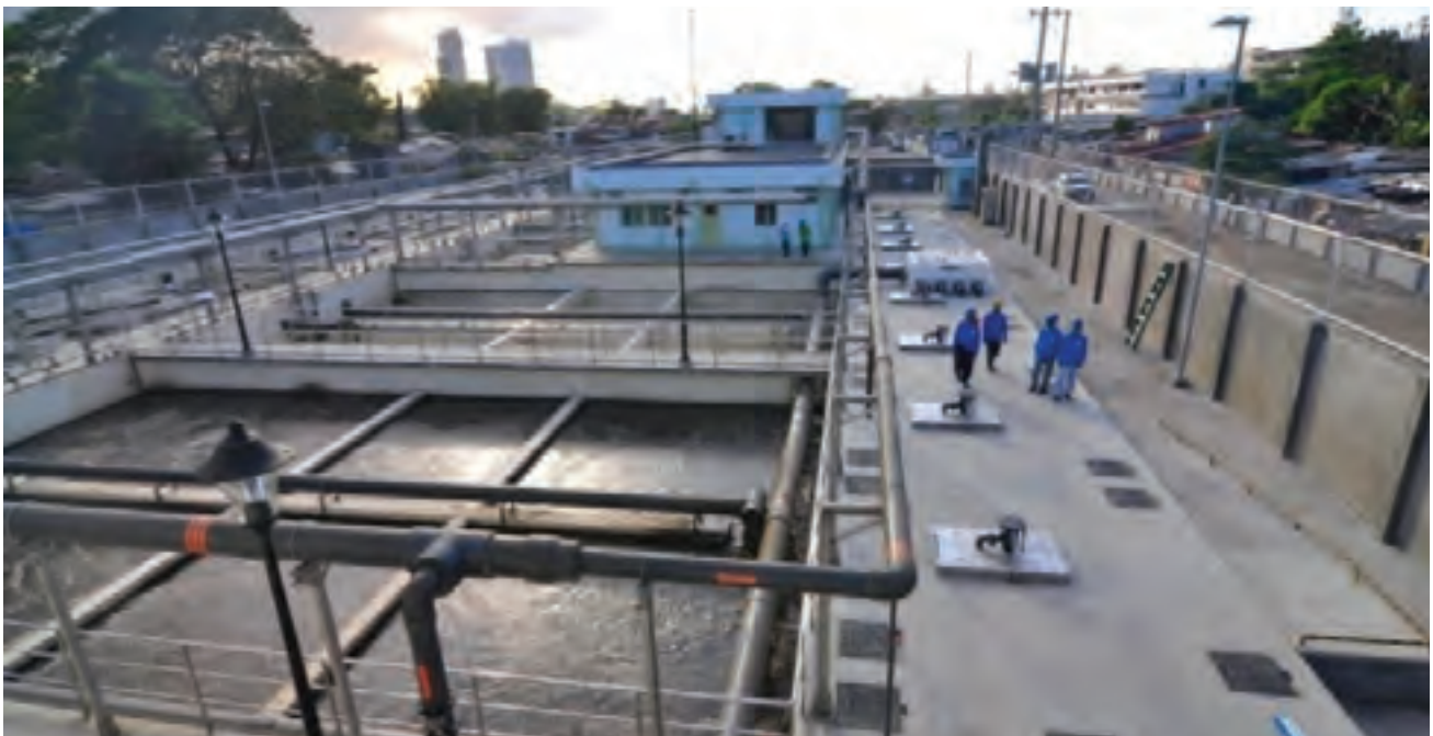
Sewage treatment plant in Singapore
