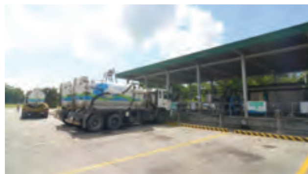
Septage treatment plant
