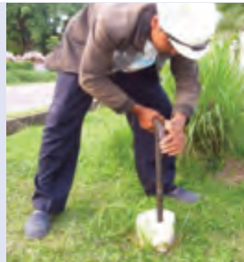
Valve turning for control of distribution
