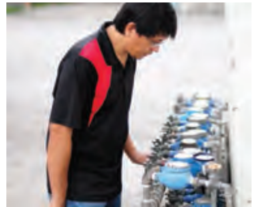
Customer water meters
