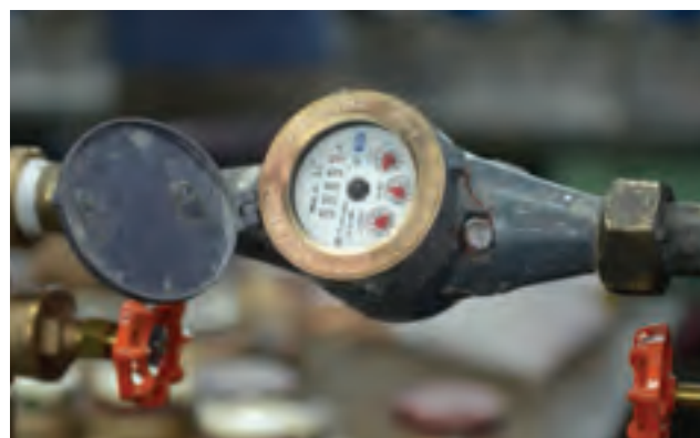
A typical MWA customer meter
