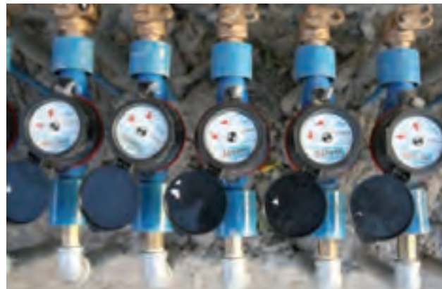
MWCI customer water meters
