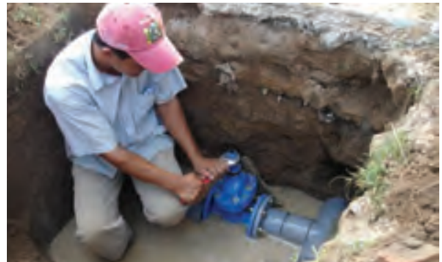
Closure valve on water network
